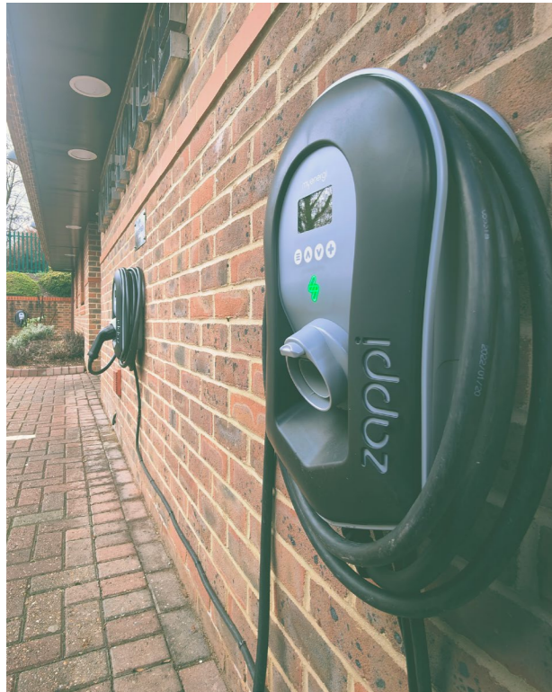
Image 09 Electric Vehicle Charging Points installed at Ashe House
